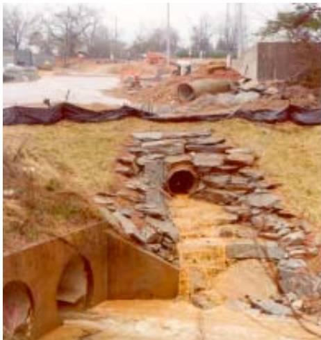
Unchecked stormwater runoff from new development
