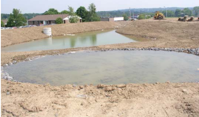
Construction and Inspection of a new stormwater management system for a new development
